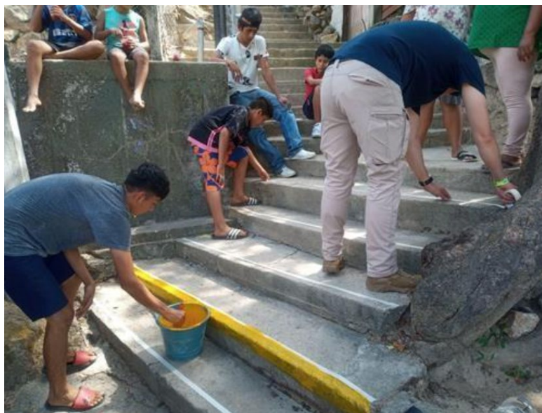
Photo 13. Safety Step Strips.
